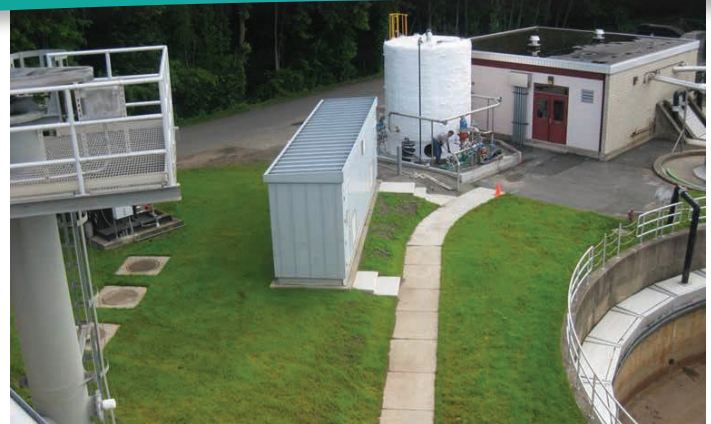
The WRRF in Ridgewood, NJ began receiving fats in 2013 for biogas production at the facility. The original 10,000-gallon capacity was expanded to 30,000 gallons.
